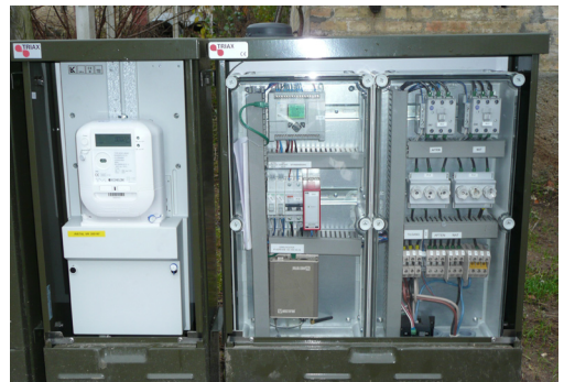
The control station cabinet holds all the streetlight equipment to control the. One station can handle up to 40 individual lights.
